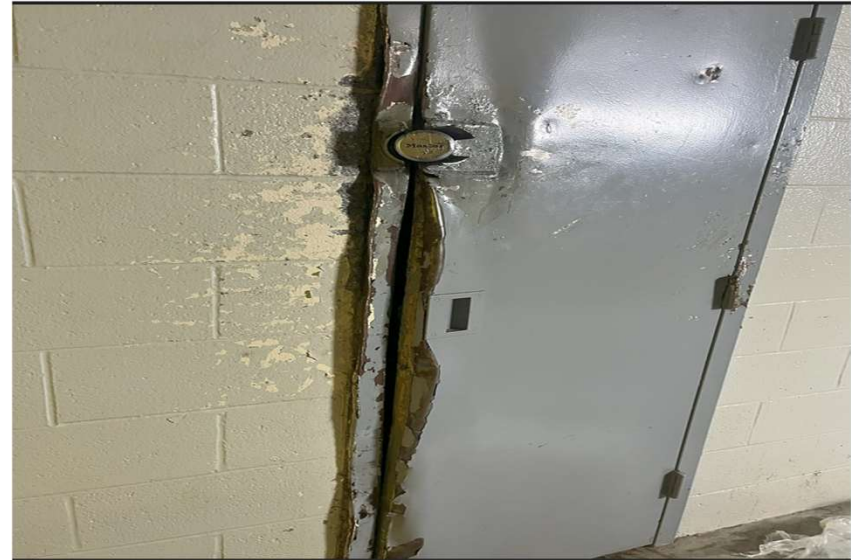
Vandalized Pipe Chase Door
