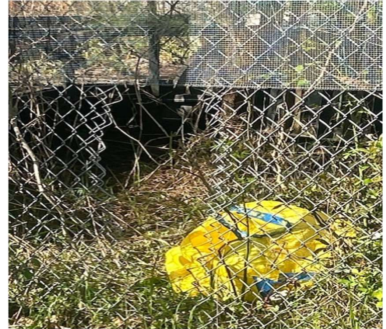
Fence Line Breach
