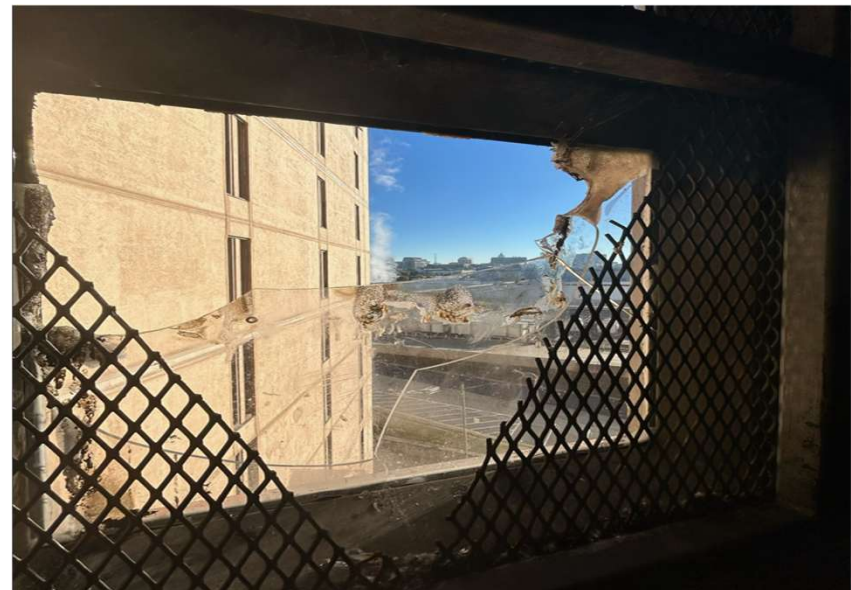
Vandalized Day Room Window
