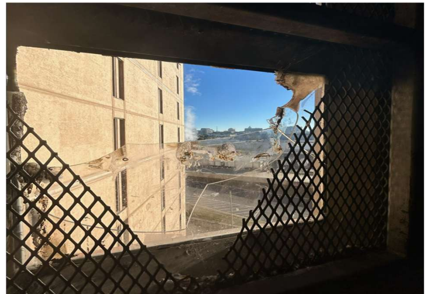
Vandalized Day Room Window
