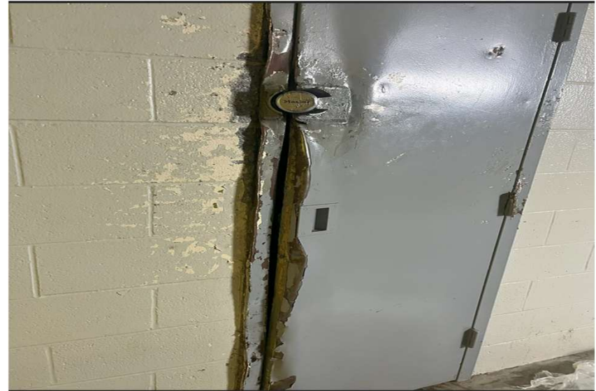
Vandalized Pipe Chase Door
