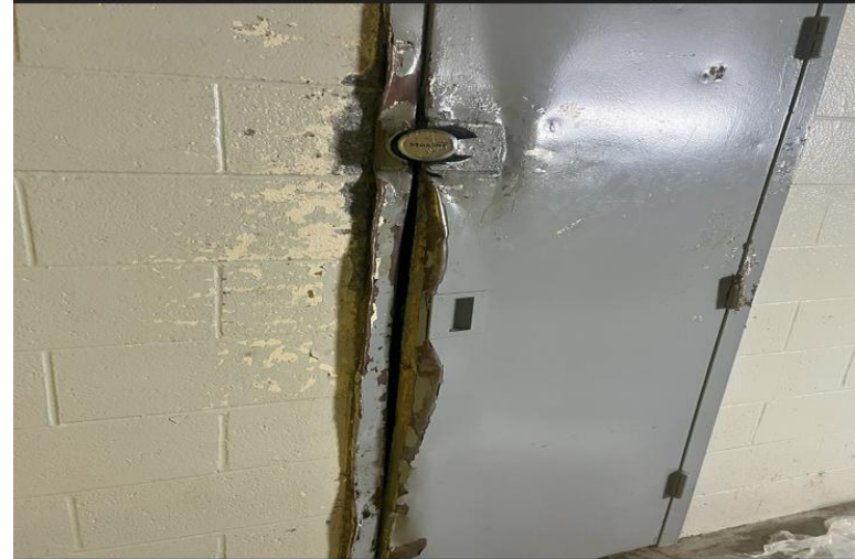
Vandalized Pipe Chase Door
