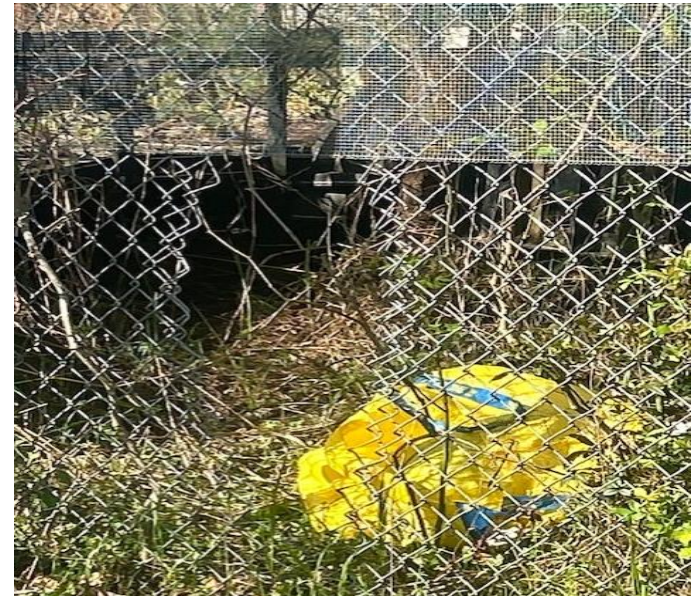
Fence Line Breach
