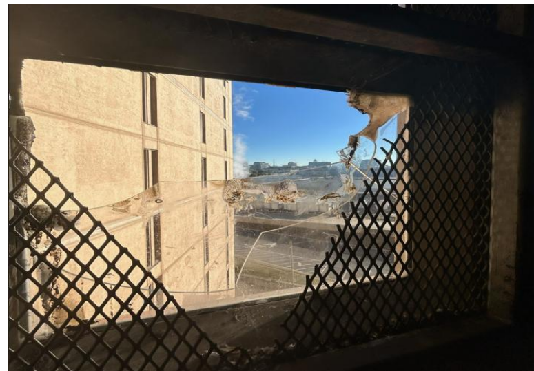
Vandalized Day Room Window
