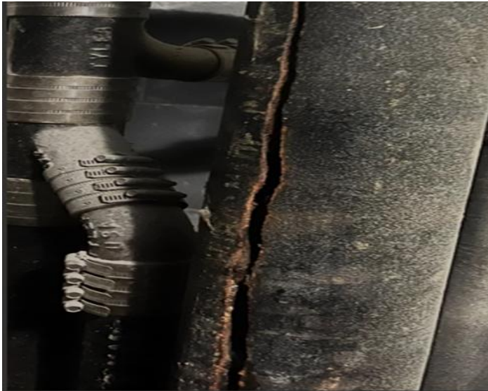
Cracked sanitary line in pipe chase
