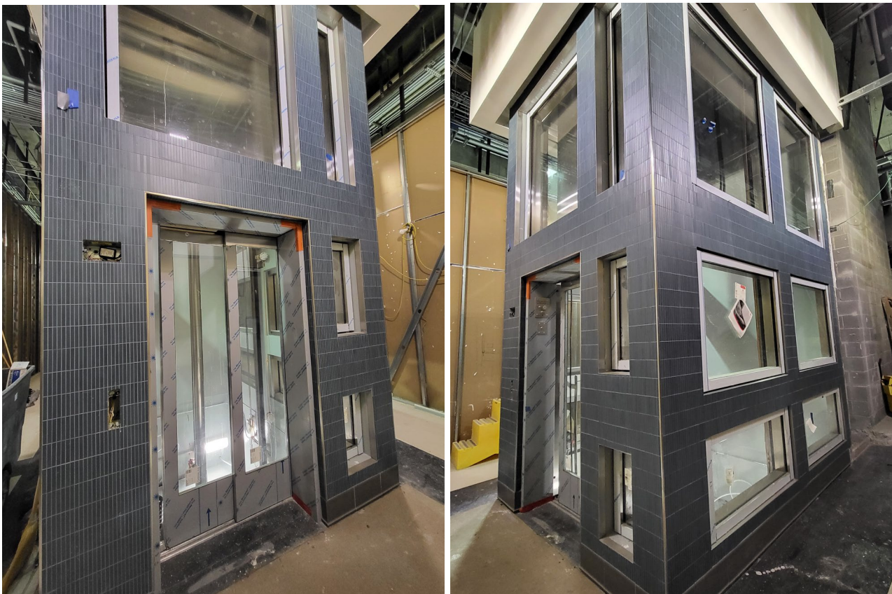
New second elevator
