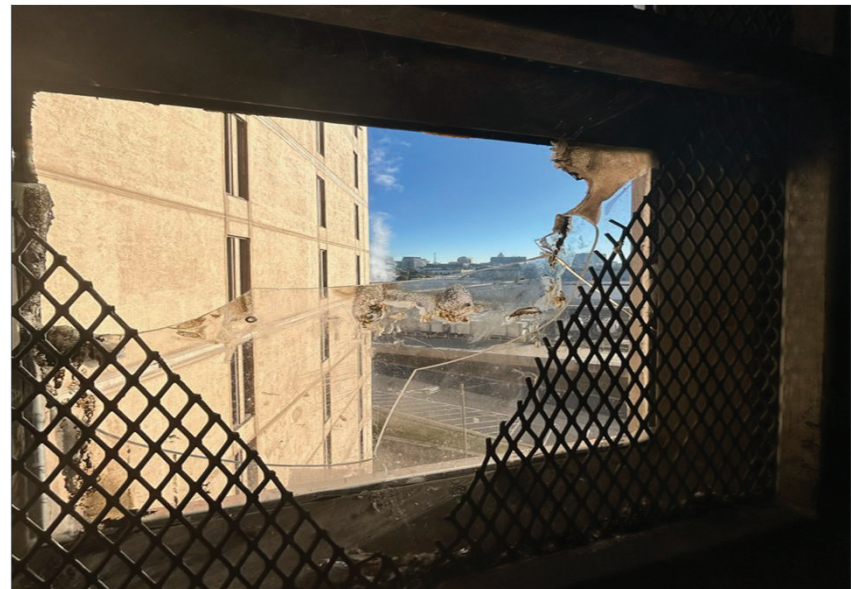
Vandalized Day Room Window
