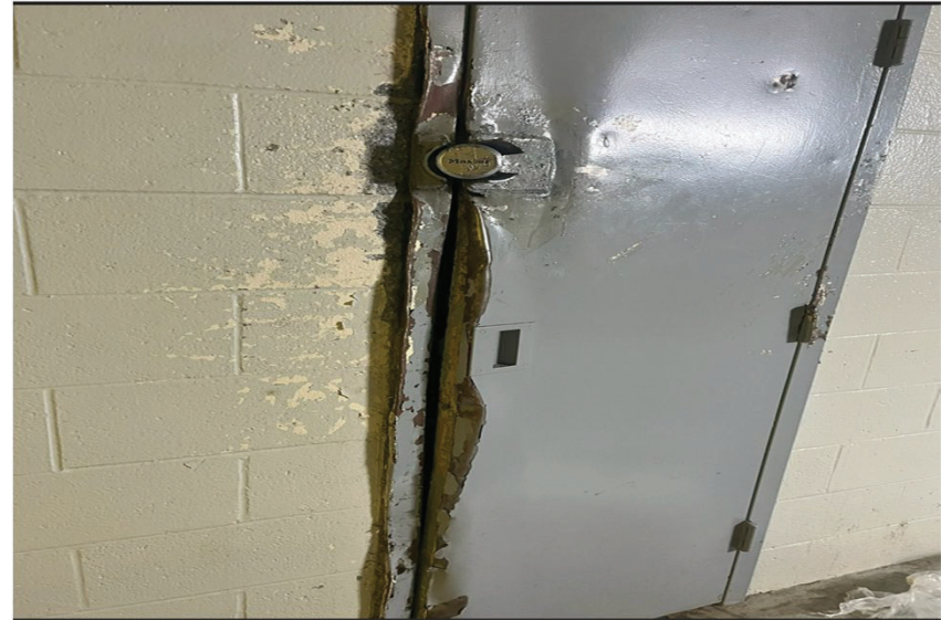
Vandalized Pipe Chase Door
