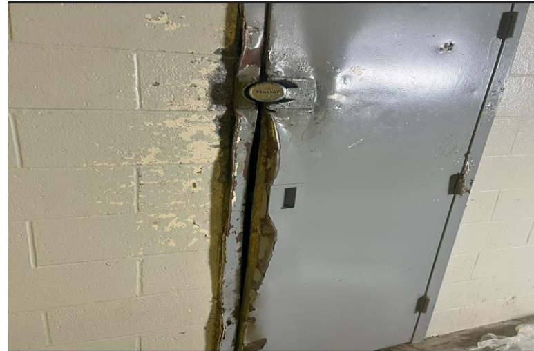
Vandalized Pipe Chase Door
