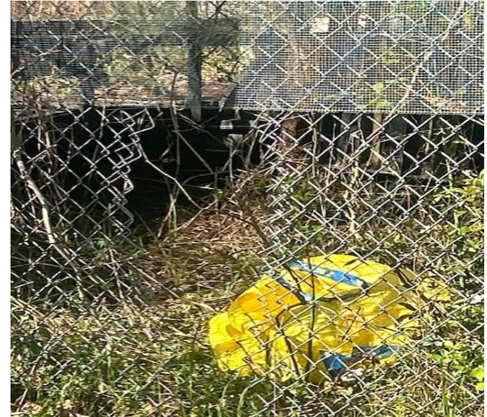
Fence Line Breach
