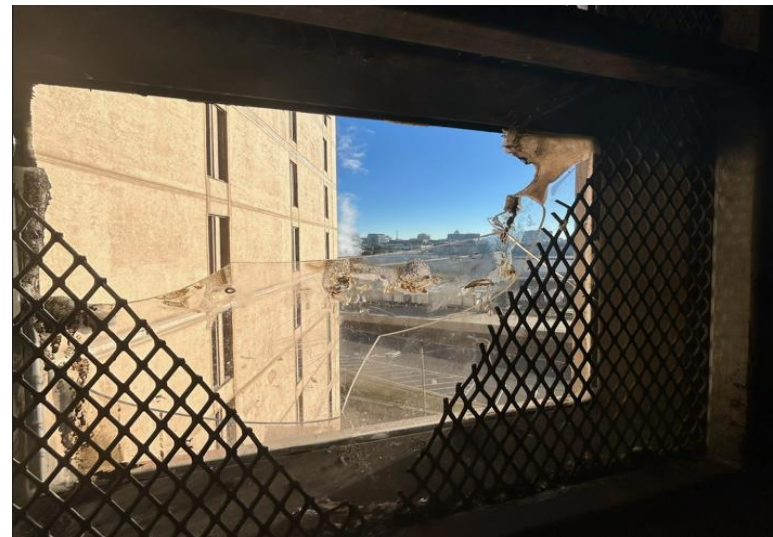
Vandalized Day Room Window
